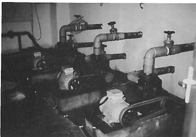
Photo 15. Seawater pumps work on a demand system and use is rotated (only one runs at a time).
