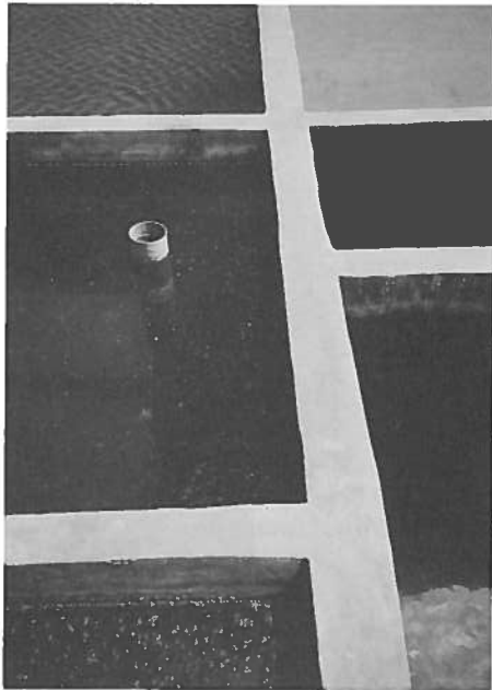
Photo 19. Close up of primary, settling, slow sand and clean water in overflow.
