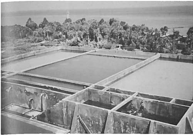
Photo 17. Cement settling tank and cement slow sand filters, primary reservoirs and overflows.
