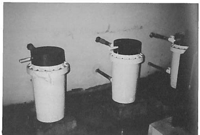
Photo 22. Diatomaceous earth filters housed inside elevated reservoir structure.
