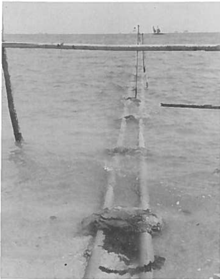
Photo 13. Two Schedule 80 3-inch PVC Intake Pipelines (one intake in shallow water and one in deeper water).
